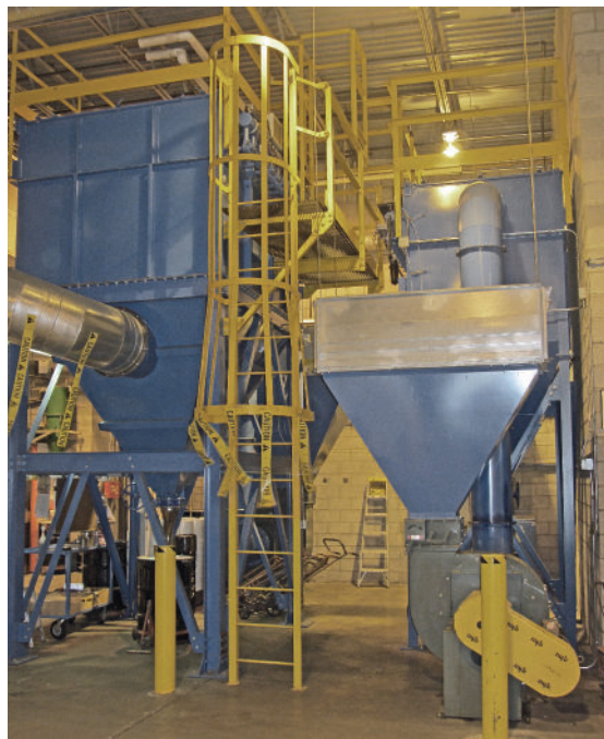
Sly's custom HEPA housing transition allowing safe recirculation of the filtered plant air.
