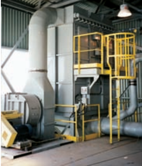
Limestone crusher and slurry mixer at a major coal-burning utility are ventilated by this TubeJet collector handling 10,000 ACFM .
