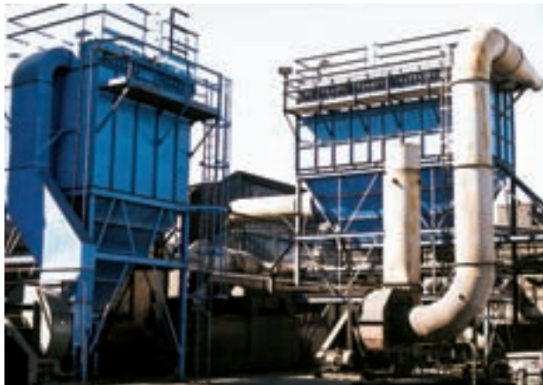
Two TubeJet collectors handle carbide dust and blast machine dust at this manufacturer. Unit at left handles 20,000 CFM; at right 60,000 CFM.
